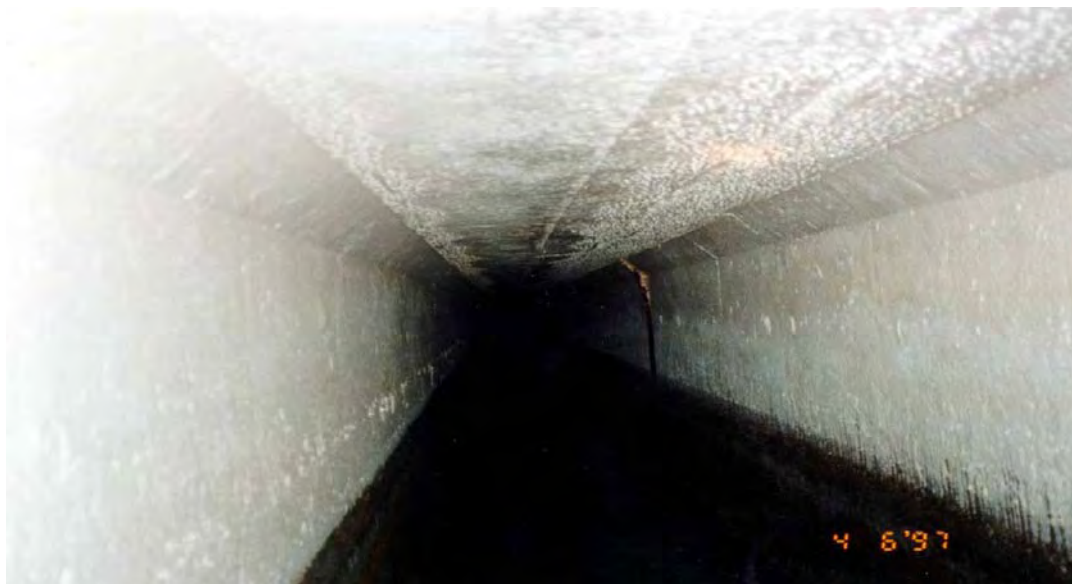
Figure 2 - Representative Picture of a Clean Sewer Line
