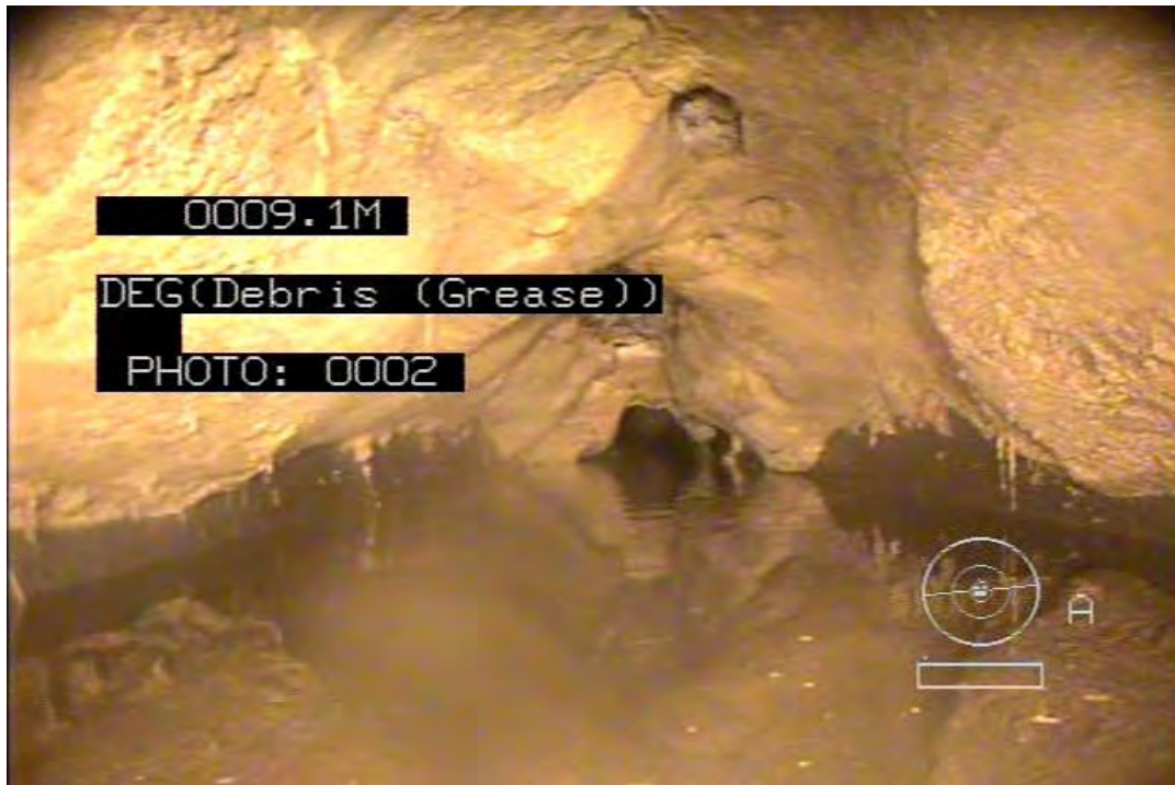
Figure 1 - Photo of the Grease Build-up in the Gilbert Trunk Line
