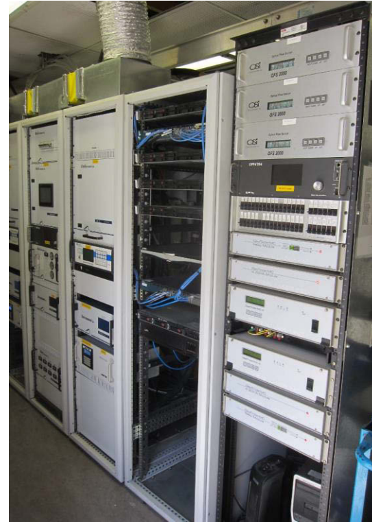
Continuous Emission Monitoring Analyzers
