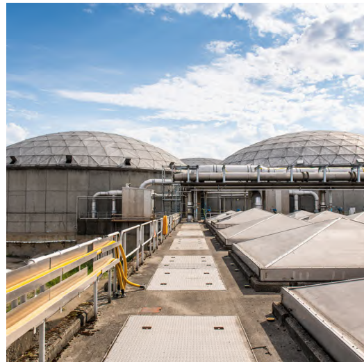
Trickling filters and solid contact tanks
