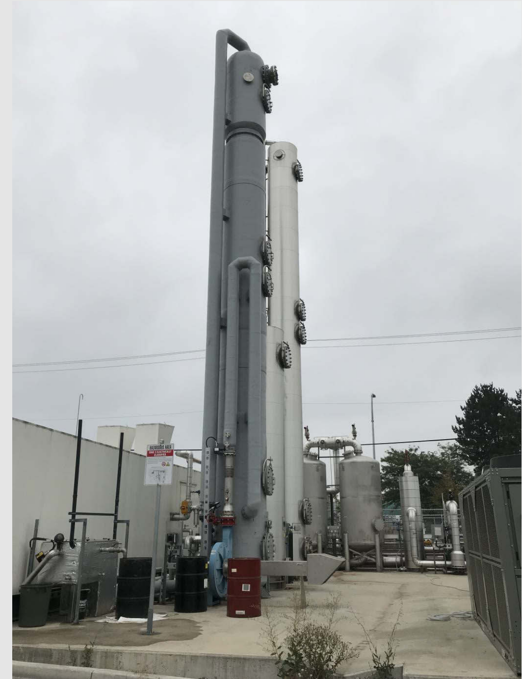
Biogas upgrade system at Surrey Biofuel Facility
