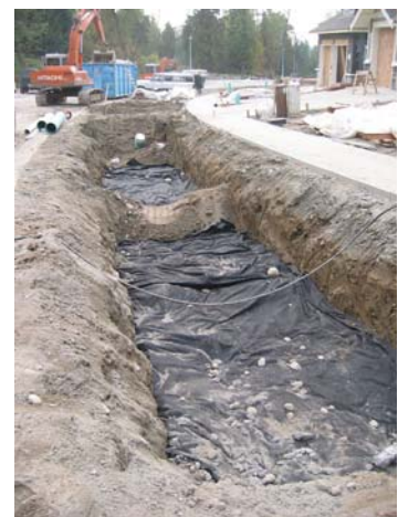
Same infiltration trench as above, before backfill, showing filter cloth wrap, and showing trench dam of native material between infiltration trench 'cells'.
