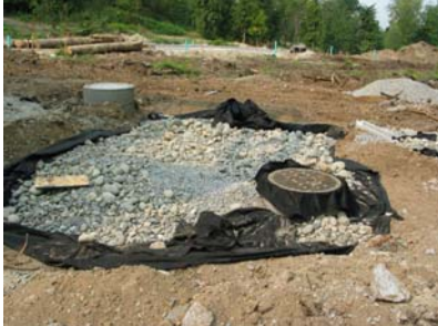
Infiltration trench with catch basin inlet at Silver Maples Subdivision in Maple Ridge, prior to surface cover with filter cloth and growing medium.
