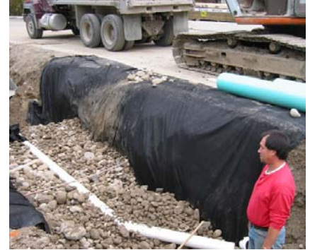
Perforated pipe over drain rock reservoir at infiltration trench under construction in Maple Ridge.
