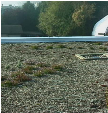
Newly planted extensive green roof showing plant-free zones at drain and edges – White Rock Operations Building
